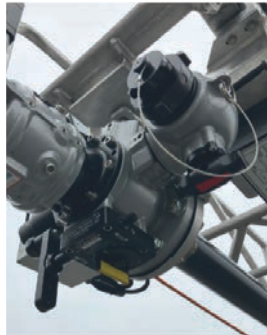
Figure 4-16. Aerial Standpipe Connection
