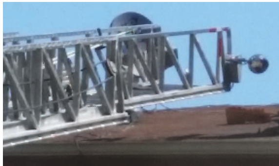
Figure 4-11. Maintain Sufficient Ladder Clearance
